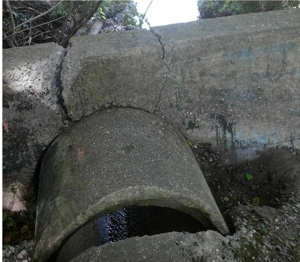
Concrete headwall is crumbling
