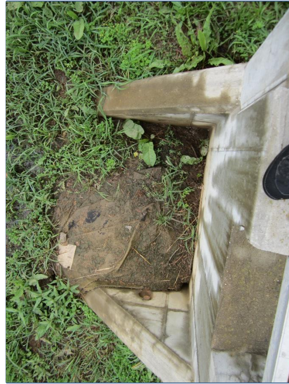
Outlet blockage by sediment
