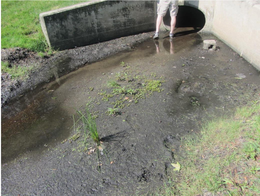
Accumulation of sediment in basin
