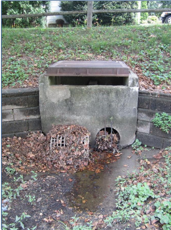
Outlet blockage by debris
