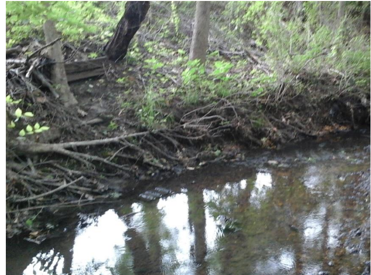
Outfall is causing scouring
